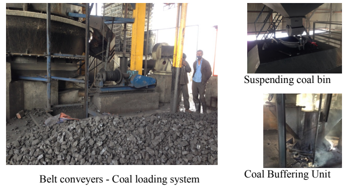
Fig. 5. Coal feeding system.
