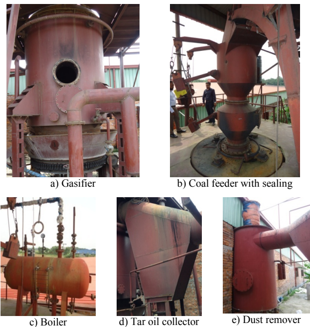
Fig. 4. Main units of gasification plant of company-1.
